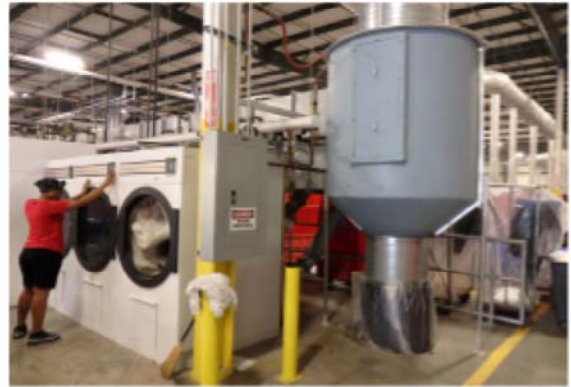
Fire Retardant Fiberglass filter with multiple dryers
