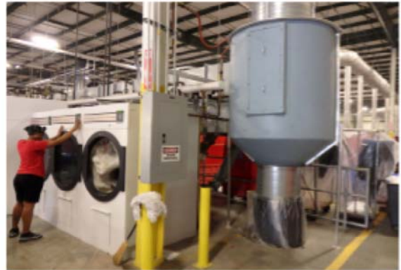
Fire Retardant Fiberglass filter with multiple dryers
